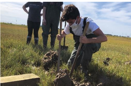
Senior Jacob Perez digs a deep hole for the new platform and osprey nest.
